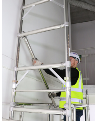
Fit a diagonal brace from the 2nd rung above the platform to the second rung of the 4 rung plain frame.
